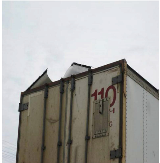
Fig. 2.39 Roof sheet—flex crack
