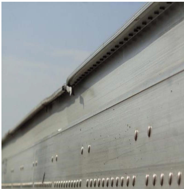
Fig. 2.21 Top rail broken
