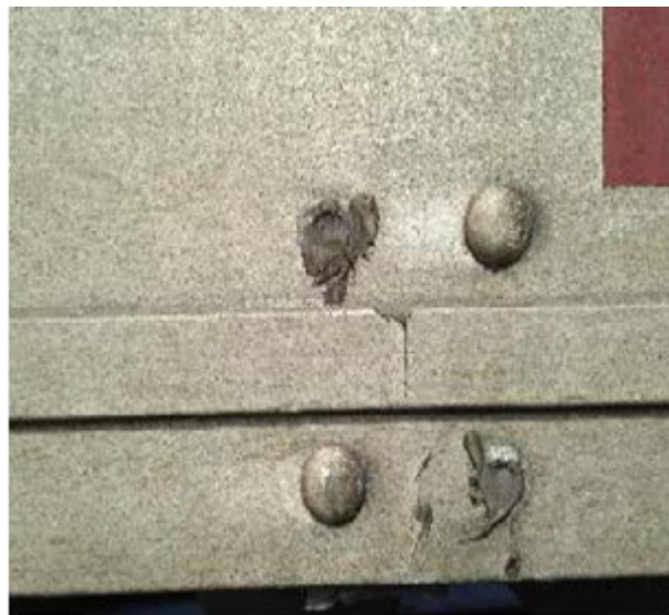
Fig. 2.11 Securement defect—broken rivets
