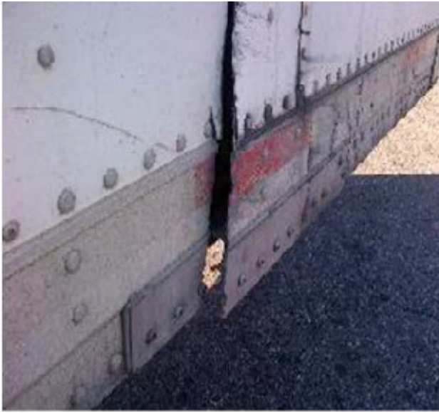
Fig. 2.4 Bottom rail break
