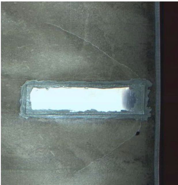
Fig. 2.40 Roof sheet—improper repair: patch material must be same as roof sheet material
