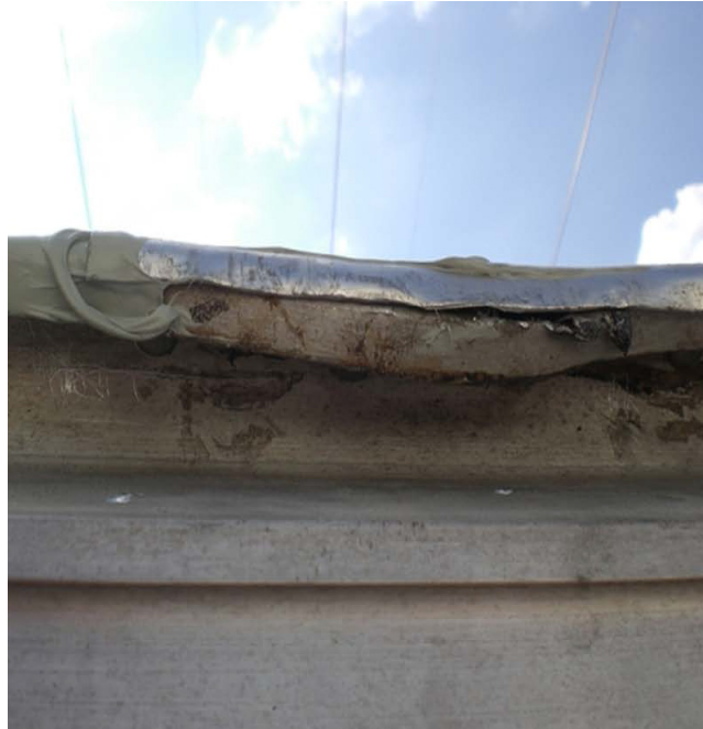
Fig. 2.20 Top rail crack
