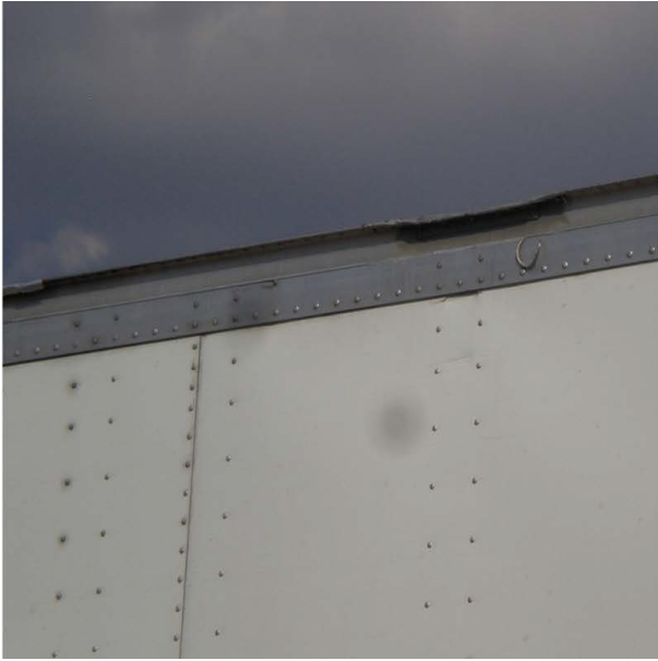
Fig. 2.23 Top rail deformation
