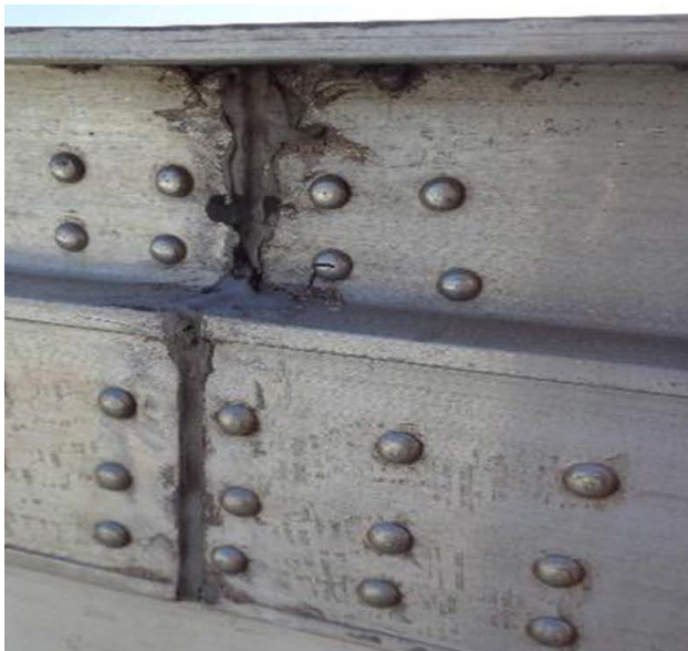
Fig. 2.25 Top rail improper repair—spliced at center
